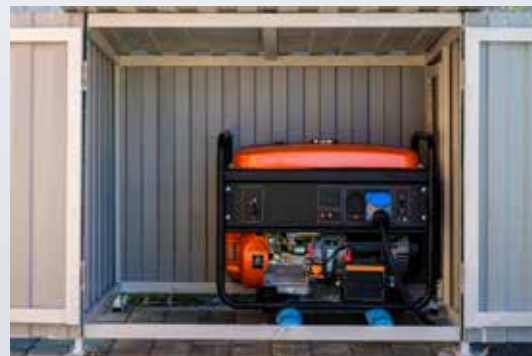
Stationärer Notstromgenerator Stationary emergency generator
